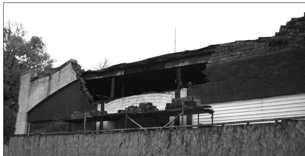
Our new Arthur Pillsbury acquisition: a warehouse in Danvers that needed some tender loving care, and a few bricks re-layed!
